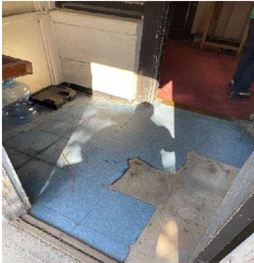
Figures 7&8: Missing floor tiles at the entrance of the office building
