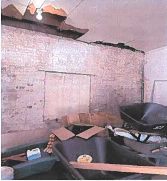
Figure 33: Garage with broken ceiling tiles
