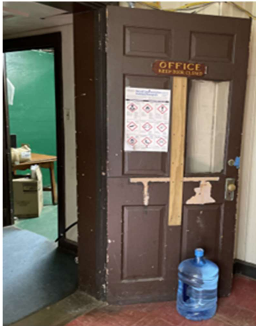
Figure 11: Broken employee breakroom door panel
