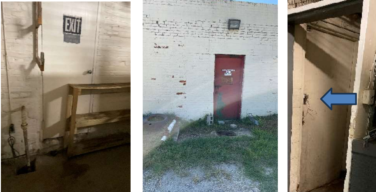
Figures 22-24: Blocked (left), padlocked (center and right) exit doors
