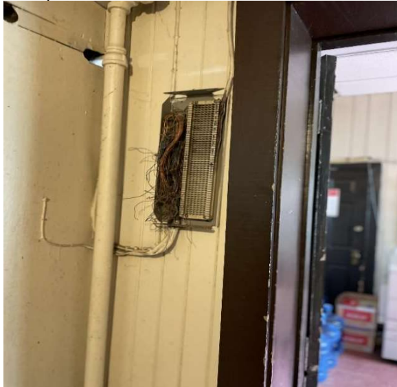
Figures 15: Wall panel with exposed wires
