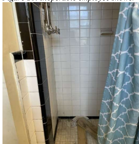
Figure 21: Inoperable employee shower
