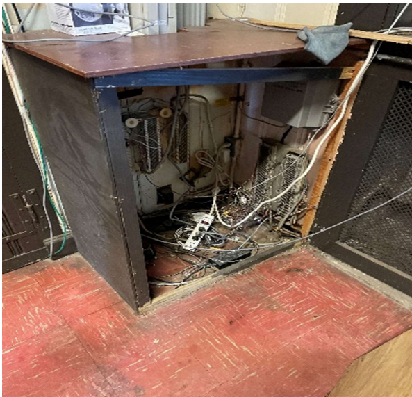
Figures 13&14: Exposed electrical wiring in the employee office
