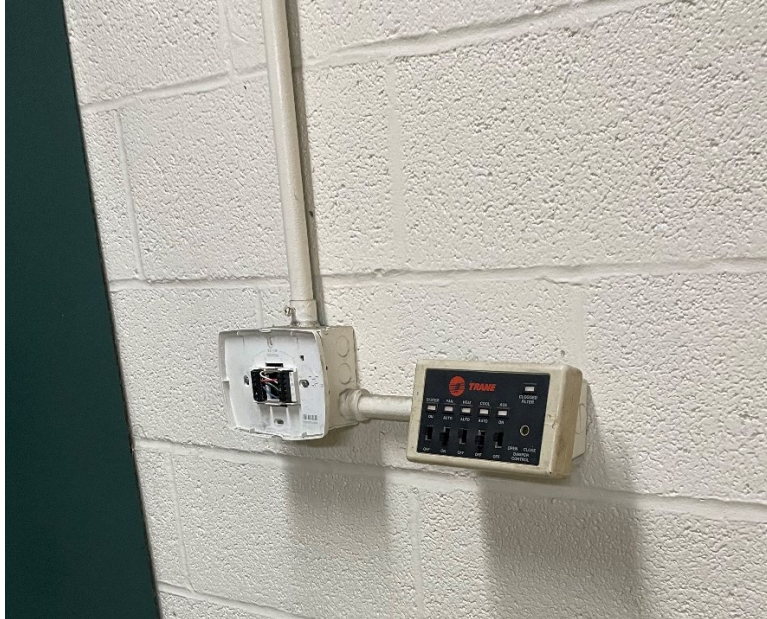
Figure 7: Locker Room Thermostat Screen Missing
