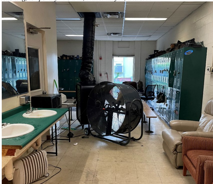
Figure 8: HVAC System not functioning, temporary A/C unit, industrial fan, and sink
