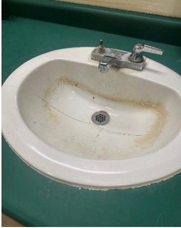
Figure 11: Before DPW improvements July 2024
