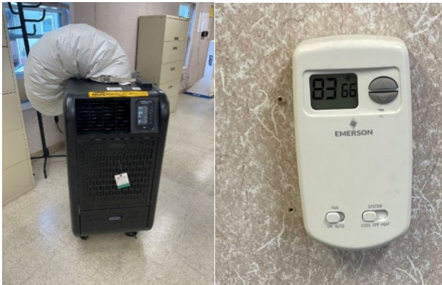
Figure 13: Before DPW improvements July 2024
