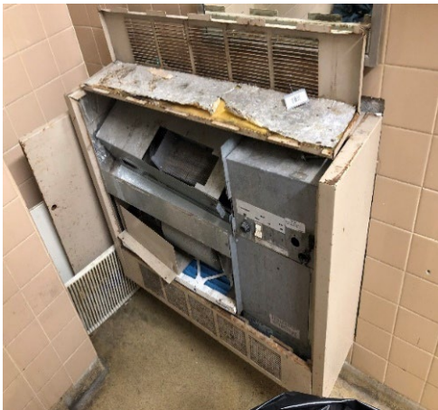
Figure 5: Before DPW improvements July 2024
