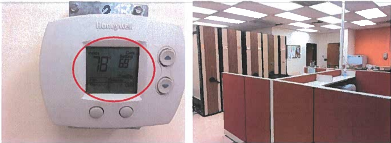
Figure 7: Room temperature higher than thermostat setting (left) and SHC staff office area where thermostat is located (right)
