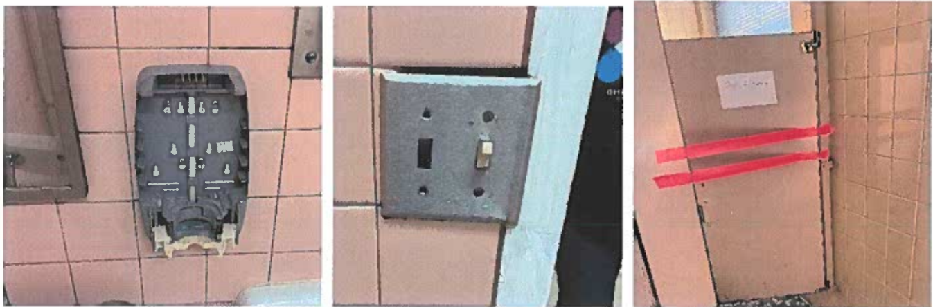
Figure 5: Maintenance issues in woman’s bathroom
