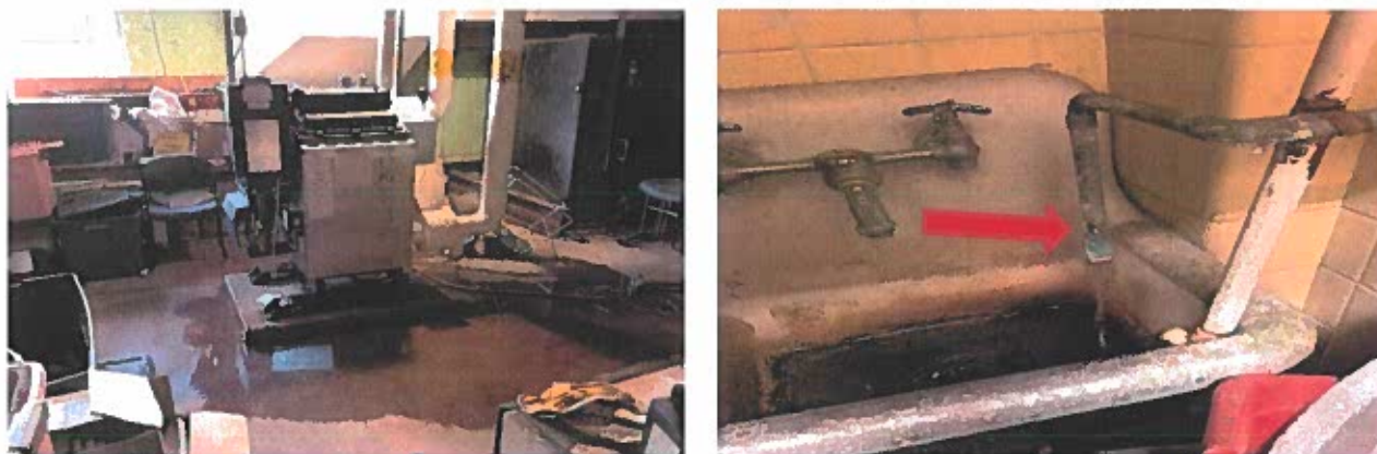
Figure 5: Water Leak in Basement (left) and running water pipe in the men's restroom closet (right).
