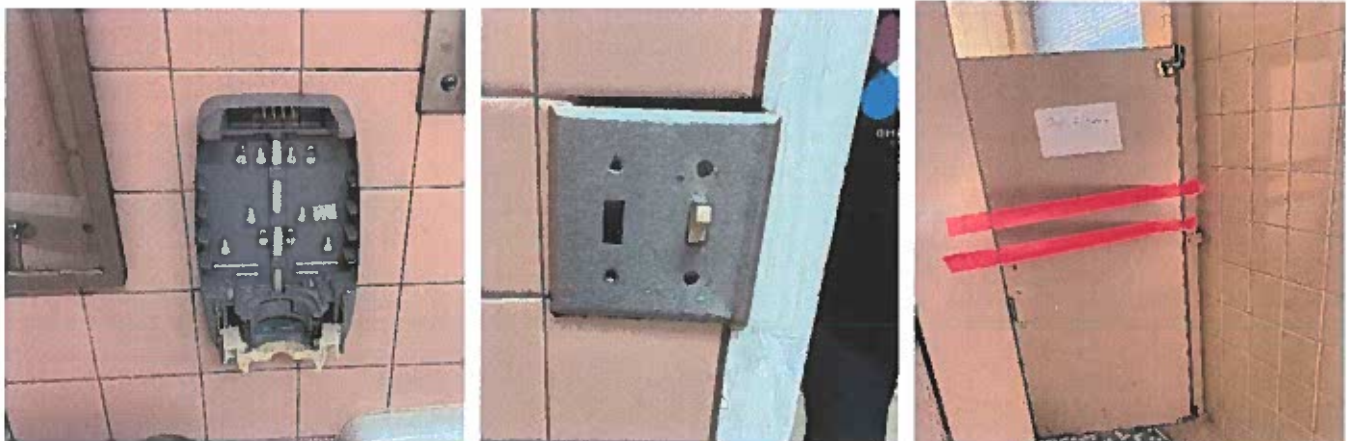
Figure 5: Maintenance issues in woman’s bathroom
