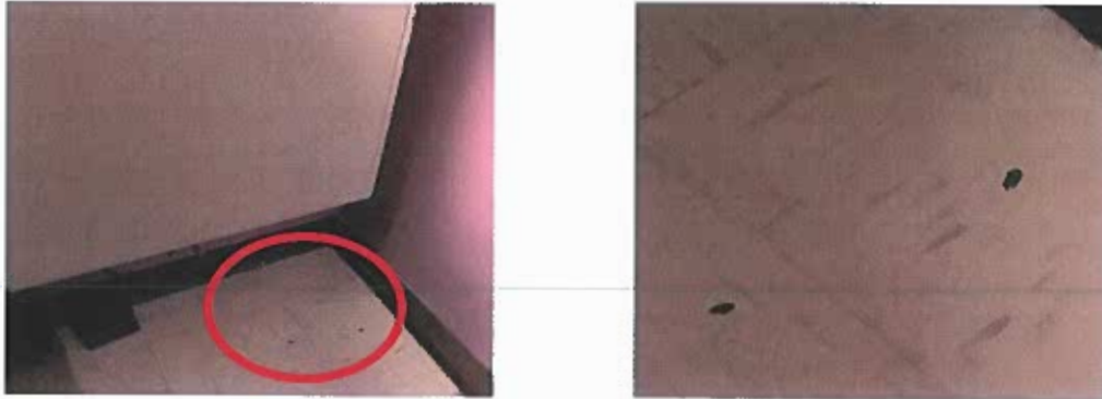
Figure 2: Potential Rodent Droppings
